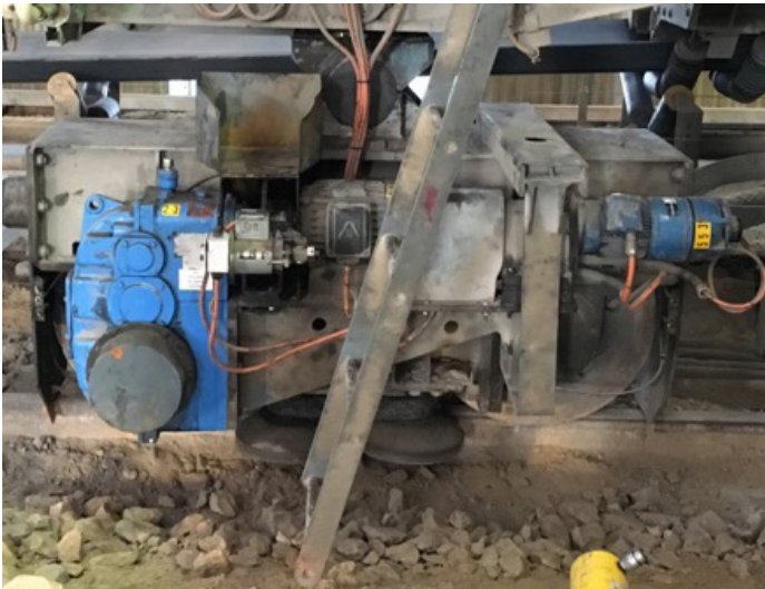
Before: An open design caused inefficiencies and required continuous maintenance.
