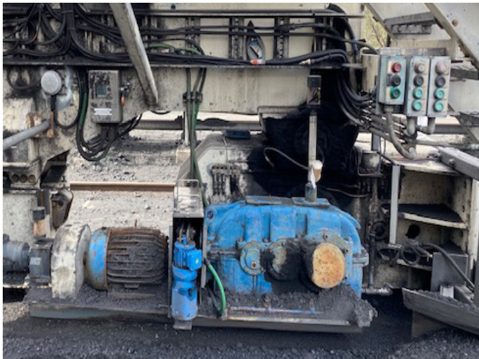
Before: Overall design and placement of equipment decreased efficiency while increasing contamination.
